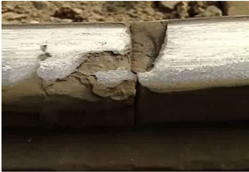
Figure Appendix M – 1 – Chipping Due to Lack of Joint Maintenance
