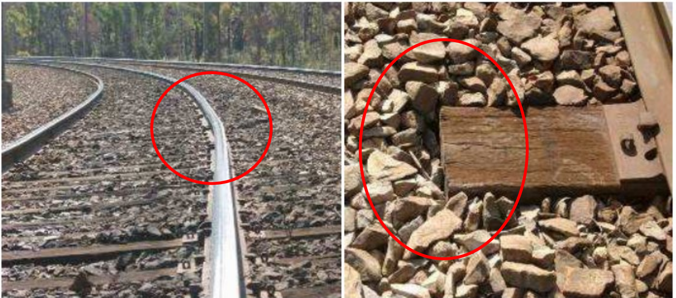
Figure SUB-PART D – 64 – Small Misalignment in Curved Track (left) and Evidence of Misalignment with Movement at Tie Ends (right)
