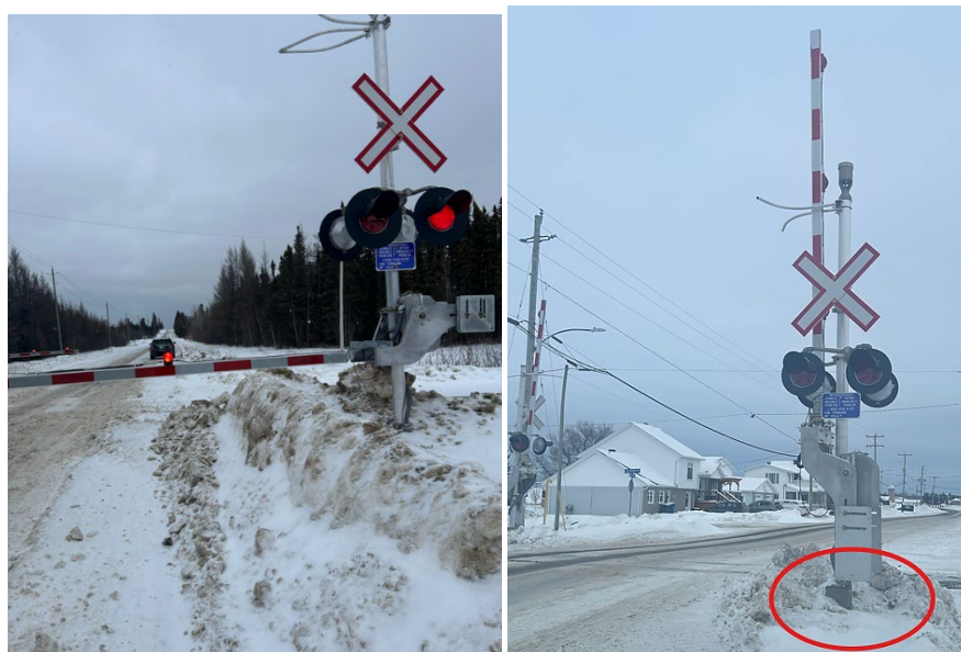
Figure SUB-PART E – 4 – Snow Beginning to Accumulate Around Warning System Gate and Counterweights
