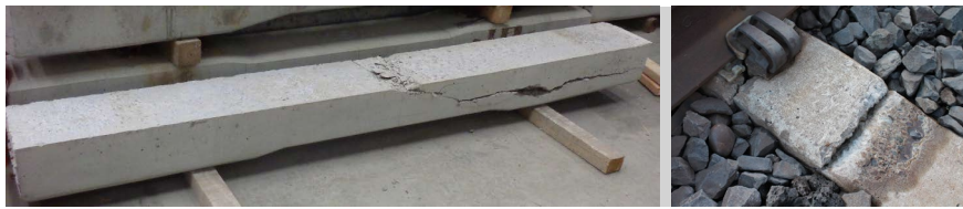
Figure SUB-PART D – 6 – Broken Through Concrete Tie (left) and Transversely Broken Concrete Tie Between Rails (right)
