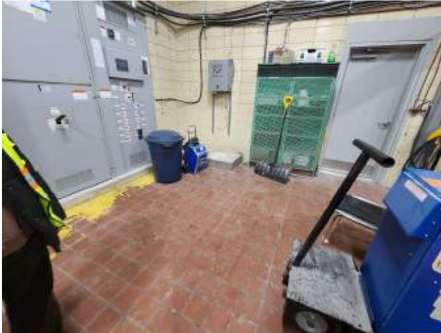
Figure 12: Battery charging area
