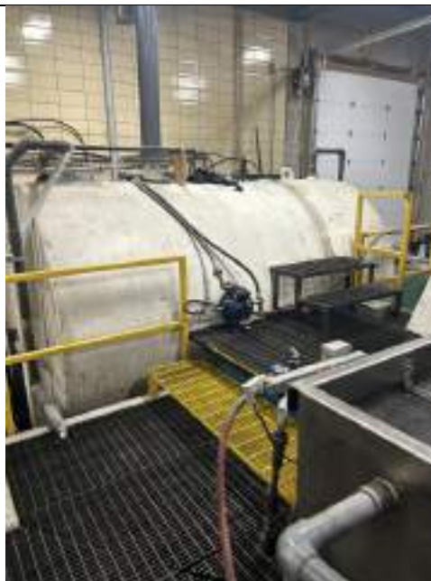
Picture 3.2 - Containment Tank
