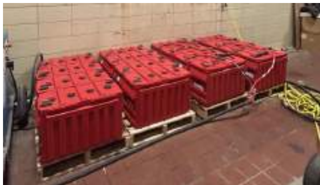
Picture 3.4 - Lead-acid batteries
