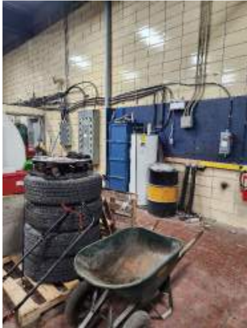
Figure 5: Cochrane Powerhouse, electrical panels and fire extinguisher
