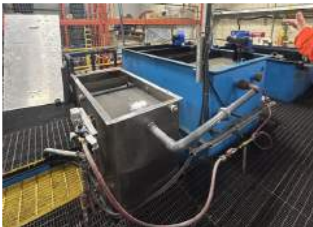
Picture 3.1 - Oil Separator
