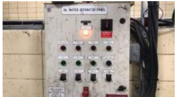
Cochrane Powerhouse - G104001
