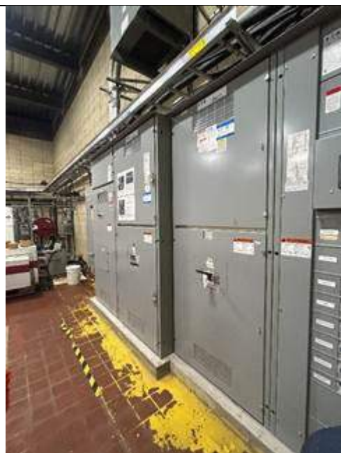
Picture 4.5 - Main Switchboard
