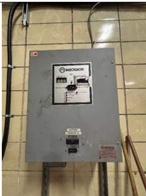
Picture 4.4 - Battery Charger B
