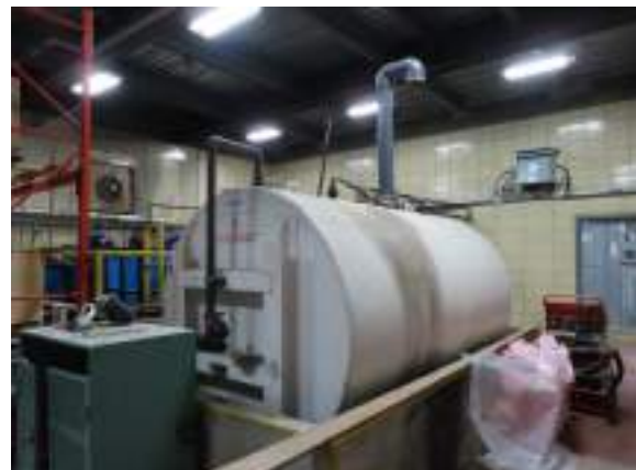
Cochrane Powerhouse - G104001
