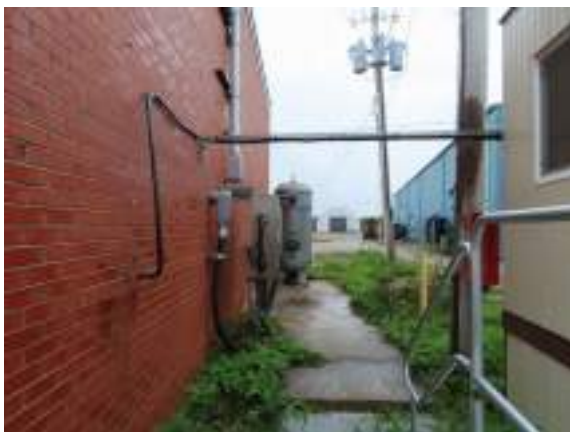
Cochrane Powerhouse - G205004
