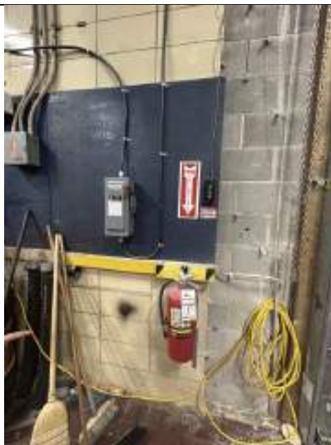
Picture 2.4 - Fire Extinguisher (Building Central)
