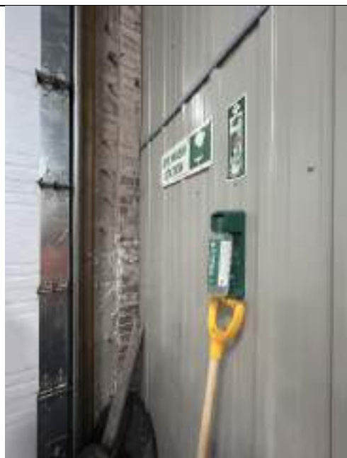
Picture 2.5 - Eyewash Station (Building North)
