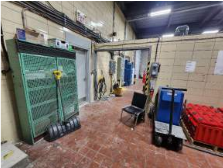
Figure 11: Battery storage area to walkway
