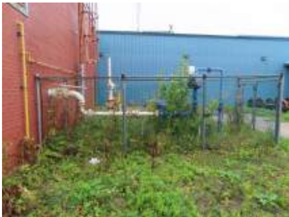
Cochrane Powerhouse - G204001
