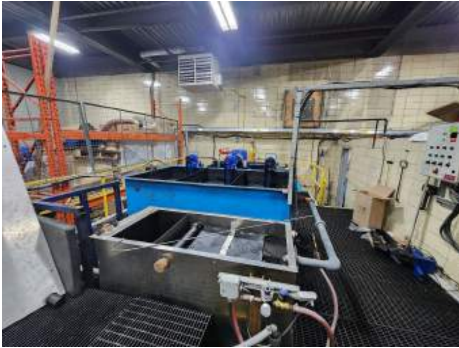
Figure 9: Oil/ water separation tanks and ventilation
