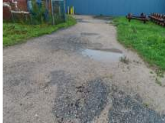
Cochrane Powerhouse - G202003
