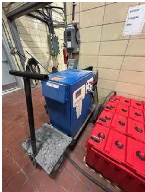
Picture 4.3 - Battery Charger
